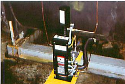
An OAM Purger installed at a 3M facility in Buffalo, N.Y.
